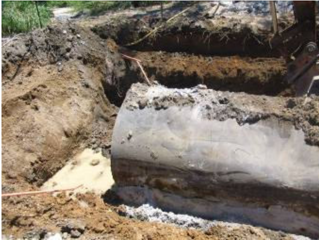
Photo 7. Underground tanks were uncovered at the former Ocean Shores Service Station site. Tanks and contaminated soil was removed from the site.
