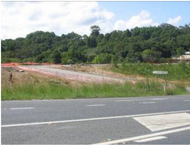
Photo 6. The Hainsville Cattle Tick Dip Site, located beside Coolamon Scenic Drive has been capped with the installation of the new road embankment at Fill 6A.
