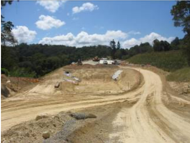
Photo 5. Because of the limited capacity to fit sediment basins beside the road footprint, a temporary sediment basin (B-F5A) has been constructed within the upgrade alignment shown here at Fill 5A.
