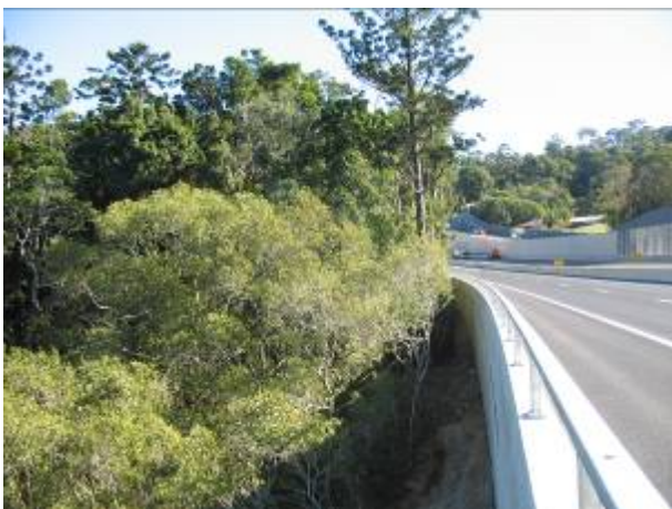
Photo 3: Completed highway upgrade adjacent to the SEPP14 wetland. The limited vegetation clearing has minimised impacts to the adjacent Brunswick Heads Nature Reserve.
