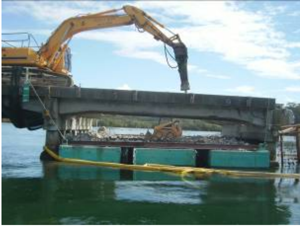
Photo 9: A catch barge located under the old bridge deck during demolition of the old Brunswick River bridge.
