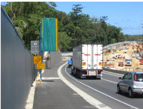
Photo 14: The permanent noise barrier wall (left hand side) near Rajah Noise is visible in this photo, and provided some noise protection while the highway traffic temporarily travelled on the new Service Road (Brunswick Valley Way).
