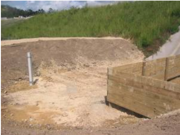
Photo 12: Detail of a typical water quality basin, used during construction as a sediment basin and in post-construction as a permanent spill basin. Photo shows an oil baffle system and low flow outlet.
