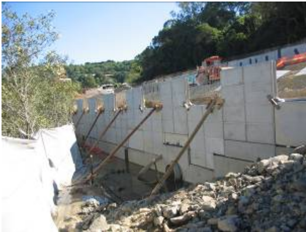
Photo 2: Impacts on the adjacent SEPP14 Coastal Wetland No 62 was minimised with the field delineation of vegetation clearing lines and a 3-metre high barrier fence. Staged removal of the 3-metre high fence was undertaken in consultation with DECC as Retaining Wall 1 was erected.
