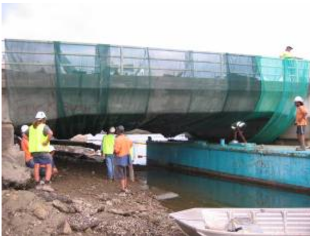
Photo 5: As part of the bat translocation plan, bat exclusion netting was placed over entire bridge spans that had been used by the bats, during staged demolition of the old bridge.
